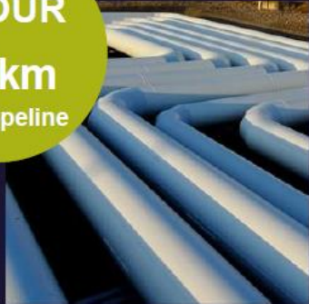
1.4m dia pipe @100bar
