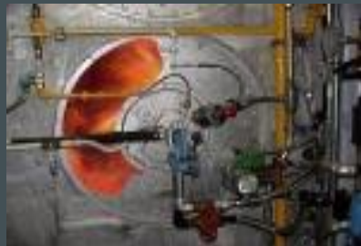
Burner Control System
